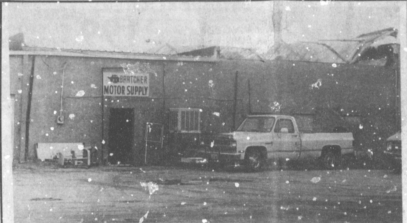
A ROLLED UP ROOF ON THURSDAY --Thursday evening, black clouds moved from north over Muleshoe depositing nearly three-fourths of an inch of rain. However, just at the beginning of the rainstorm, heavy winds drew the cloud into town. One victim of the storm was the roof of Bratcher Motor Company, which rolled up due to the intense windstorm. No other measurable damage was reported due to the storm. Intermittent rain fell all day on Friday, and as evening approached, black clouds were again rolling in from the north. (Journal Photo)
