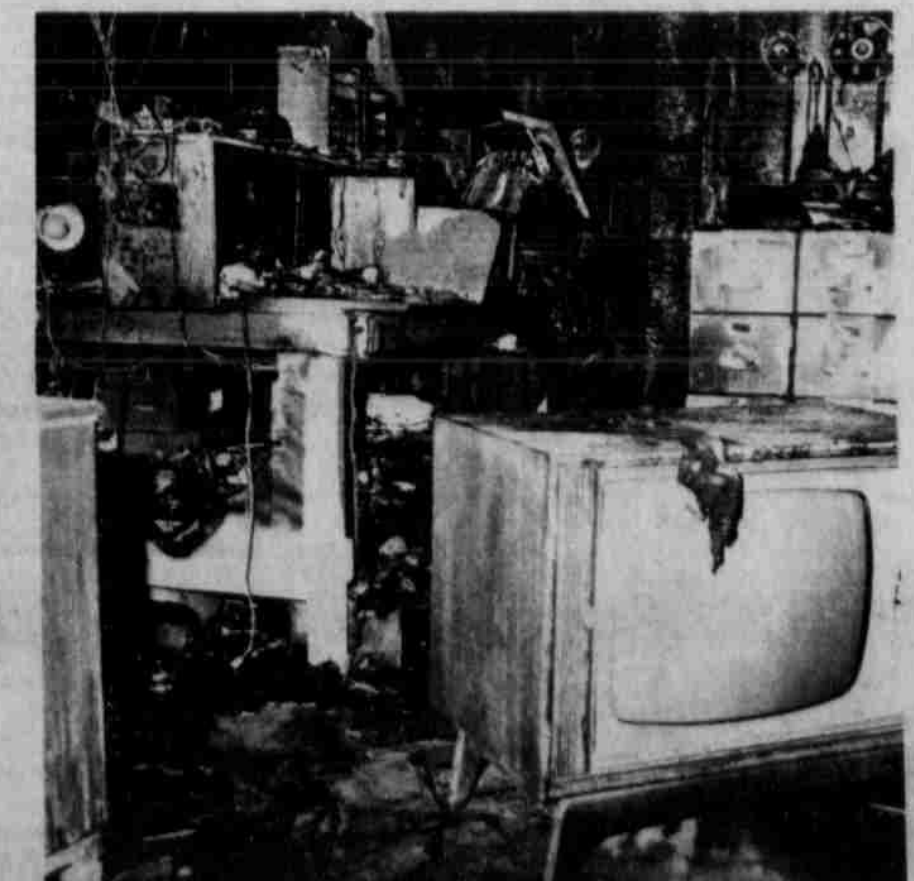
FIRE GUTTED Volunteer Fire Chief Leon Durham's business TV Corner in the early hours Tuesday morning. Approximately $17,000 damages are estimated in the fire that officers say was an act of arson. This shows a portion of the damage to the interior of the building. (Staff Photo)
