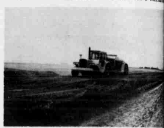
THESE ARE parallel terraces constructed on the Dan Jones farm southeast of Littlefield. Jones installed part of the terraces this spring and plans more this fall. (S. Photo)
