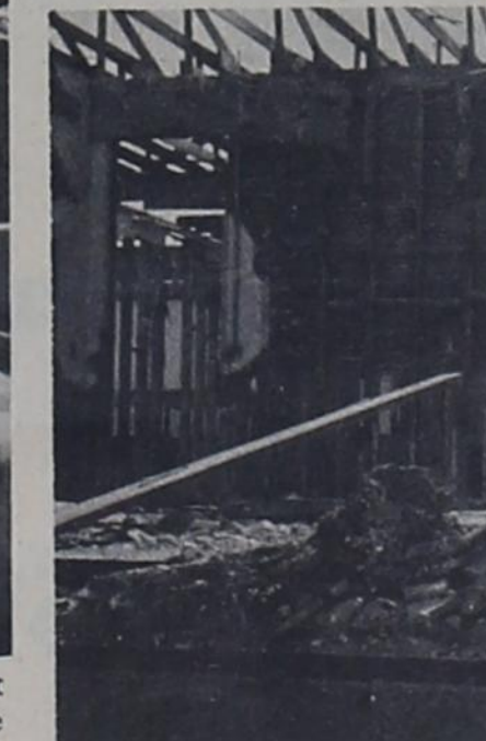
WRECKING CREW AT WORK -- Jim Pierce, high school principal at Texico school, is heading the work of wrecking the old Texico School building which was condemned several years ago. The crew has been making good progress since the operation began two weeks ago. Pierce, left, stated that he hopes the wrecking work will be completed in another two weeks.
