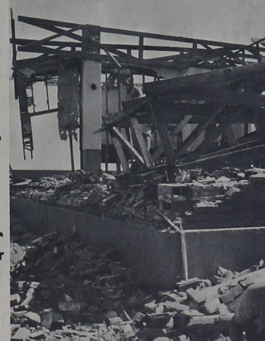
IF ONLY BRICKS COULD TALK -- Then these bricks torn out of the old Texico School building, erected in 1918, would have many a tale to tell. About all that remains of the once proud building is a pile of rubble. Crews are making good progress in wrecking the building. Bricks are being sold and hauled away almost as fast as they are torn down. When the wrecking work is completed the ground will be levelled and made ready for the beginning of school and hopefully a new building in the not too distant future.
