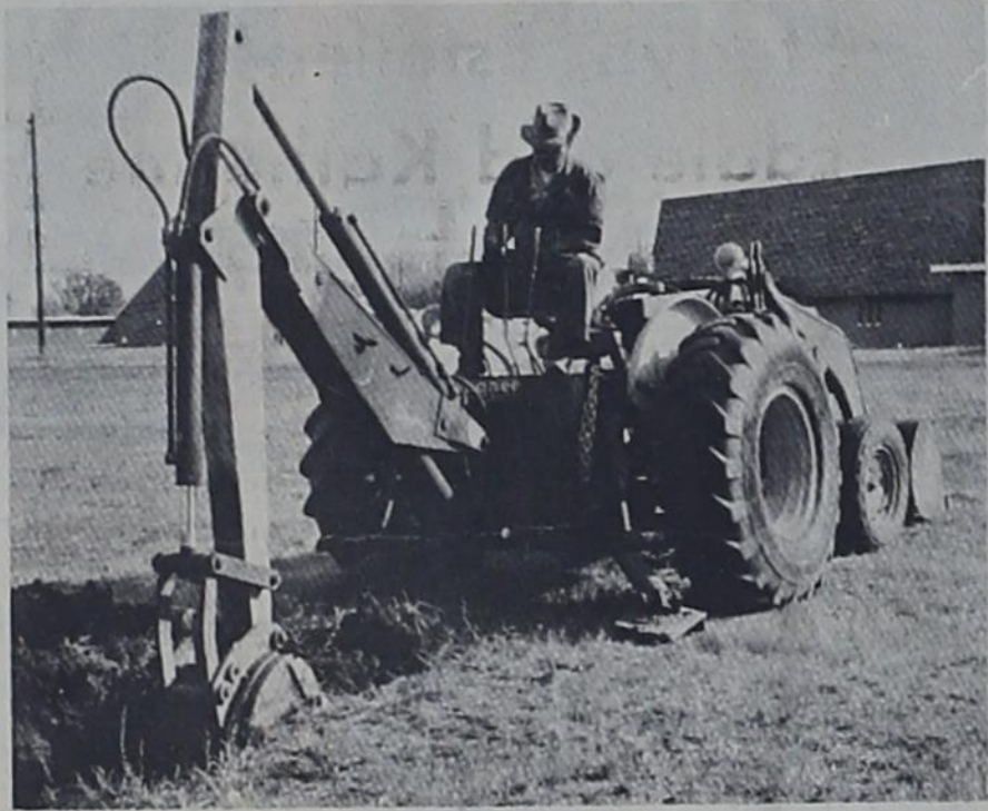
THIS IS THE WAY we dig the holes and ditches for new water lines in 1967, said Venable who related that he had dug many a "ditch" and many holes to unclog sewer lines with nothing more than a pick and shovel.
