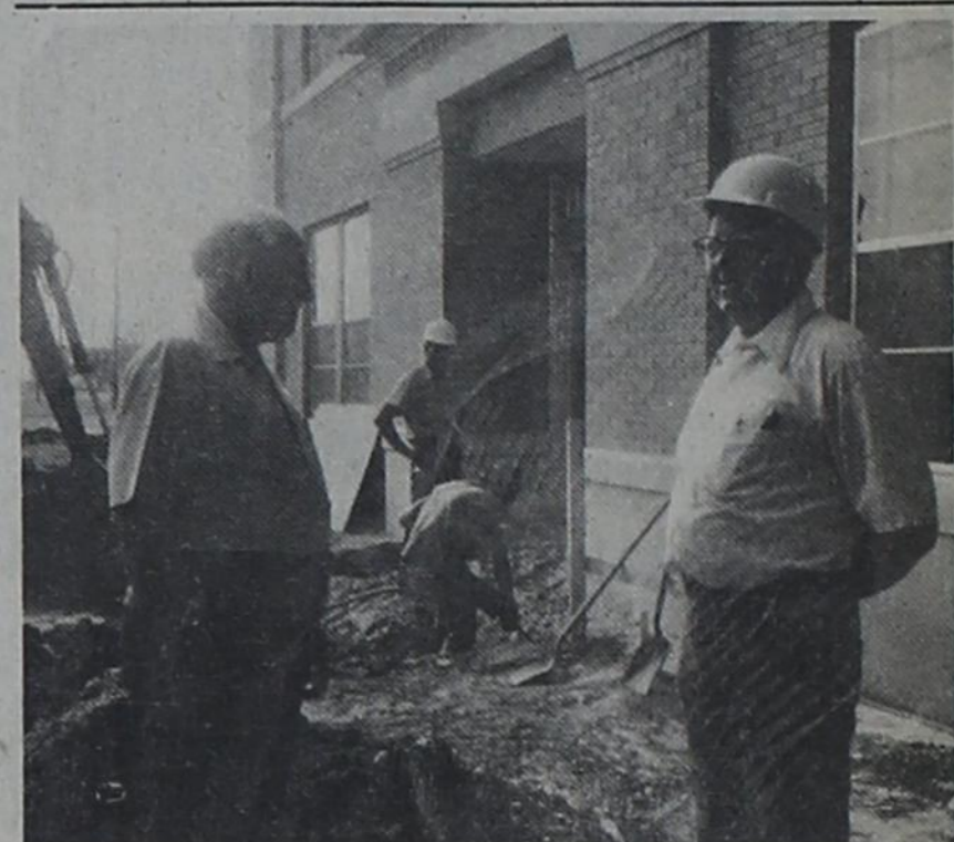
CONSTRUCTION BEGINS -- Construction on the new Parmer County Law Enforcement Center has begun with the clearing of trees from the north side of the Court House and the elimination of cement steps and sidewalk from the north Court House entrance. As the construction men work in the background, County Judge Archie Tarter, left, discusses the work with construction superintendent, Harold K. Haynie of Farwell. The contract for construction of the facility will allow 260 working days for completion. John C. Cornell, Inc. was awarded the bid in the amount of $277,715.
