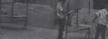
Rose Drug and Gift Shop will be one of the most modern drug stores in the area when the remodeling and repair work is completed. The project is under direction of Charlie Hromas, local building contractor. The front of the store is undergoing a complete face lifting and the interior will also be remodeled.
