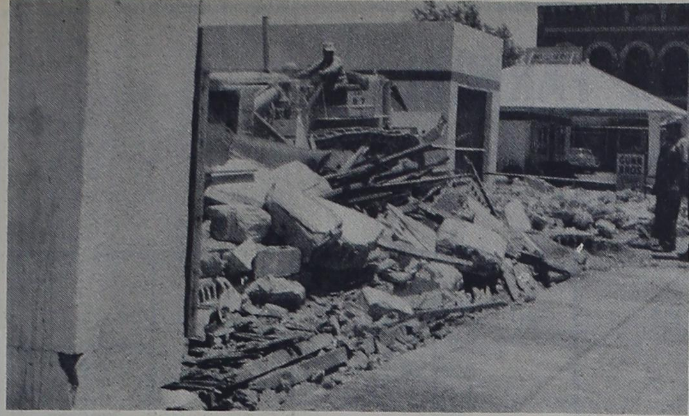
Causing much speculation on Tuesday was the razing of the old variety store building in Texico. Many town residents gathered to watch the wrecking crew at work and speculate on what would be built in the location. Owners of the property, Citizens Bank of Clovis, had no comment to make on what would be erected on the location but said the space was not needed for parking purposes. All remnants of the building had been removed from the property by middle of the afternoon.
