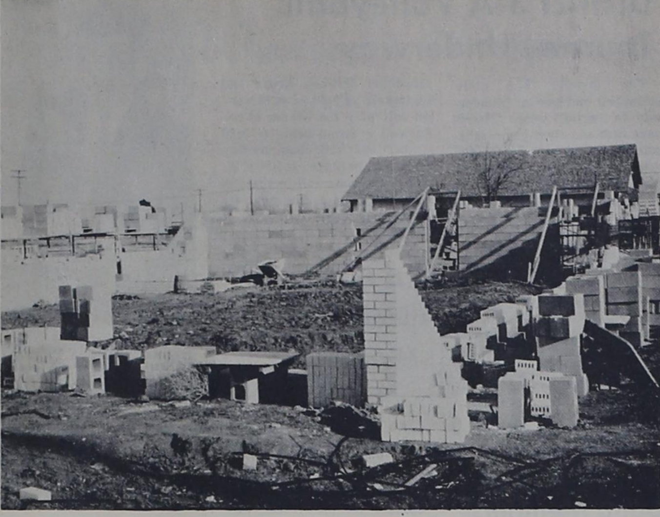
Materials have been moved onto the ground and work has begun on erecting the walls at the Texico Branch of Citizens Bank. The structure is expected to be completed in approximately 90 days.
