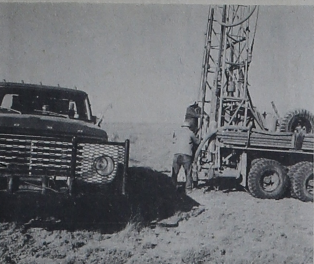
CORE DRILLING at Catfish Draw just north of Bovina is being done this week by employees of Parmer County Soil Conservation Service for the purpose of determining the soil formation under the damsite at the Running Water Draw Watershed, determining what kind of soil is in the spillway that is to be cut and determining where the best material is for building the earthen dam.
