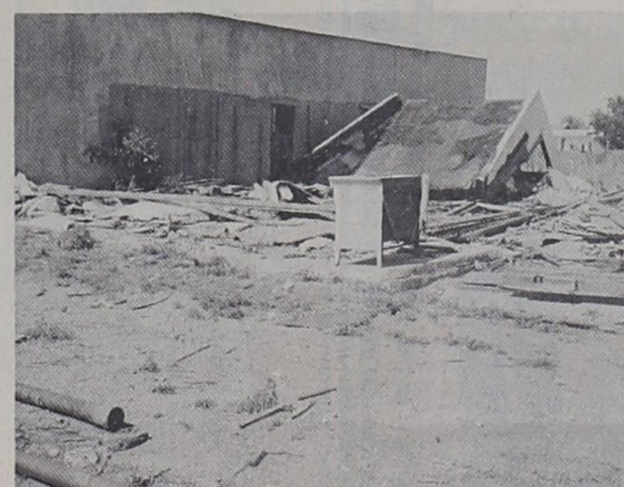
Clearing away of old buildings in Texico continued this week with the tearing down of the "old telephone office" which was built in 1906. The building was used continuously as a telephone office until the local operator service was discontinued in 1942. After that time it was used as a home by Mrs. Jim Moore, who operated a cafe in Texico for a number of years. She recently sold the property to A. W. Skarda of Clovis. Remains of the building are shown.
