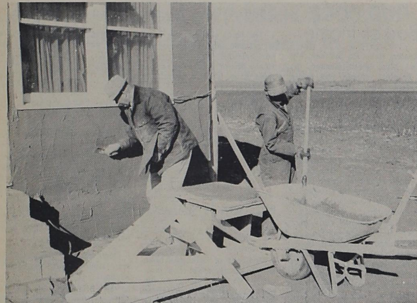
Some folks worked during the Christmas - New Years Day holiday week. Zeferino Villarreal (right at wheelbarrow) makes his home ready for the winter with the help of Clyde Meador, plasterer from Clovis. The home is located on the Joe Schilling farm in the Oklahoma Lane community.
