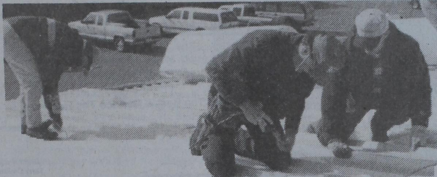
When the Farwell Community Center needed a new roof -- the Rotary Club volunteered its time and expertise to do the job. Jimmie Mace spearheaded this project.
