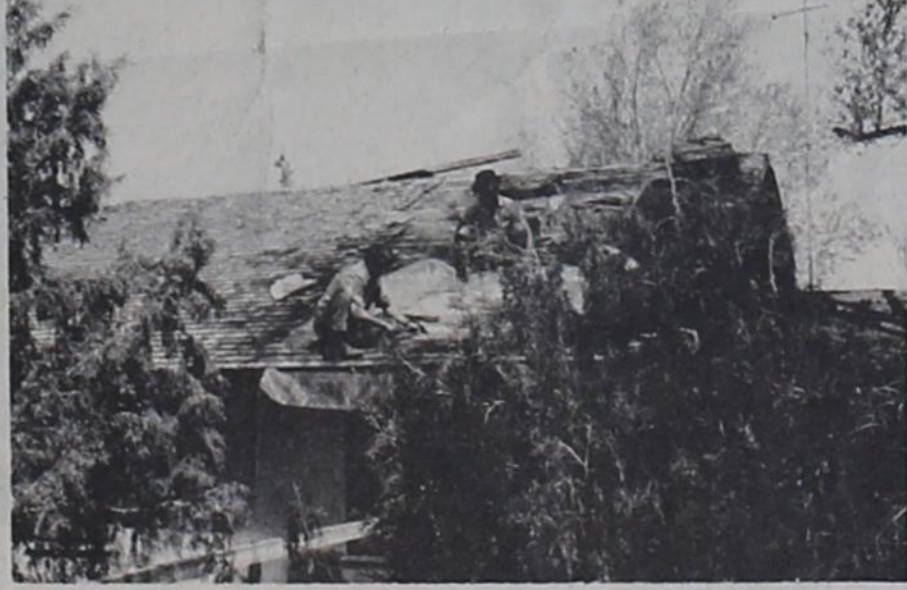
STORM DAMAGED ROOF -- Workmen are busy repairing the roof of the Charles Bradley home southwest of Texico which was heavily damaged by an apparent tornado or twister last Thursday evening. The winds blew the roof from the southeast corner of the home and the rain caused the ceiling to collapse. No one was injured as Bradley was able to get his family to a basement before the storm hit. A fence at the home was also damaged and many trees were uprooted in the area.
