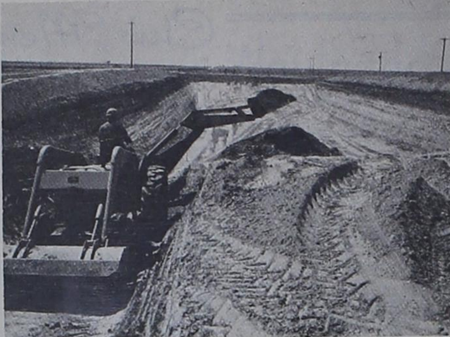
Tailwater recovery pit being completed on the Lester Norton farm four miles north of Farwell.
