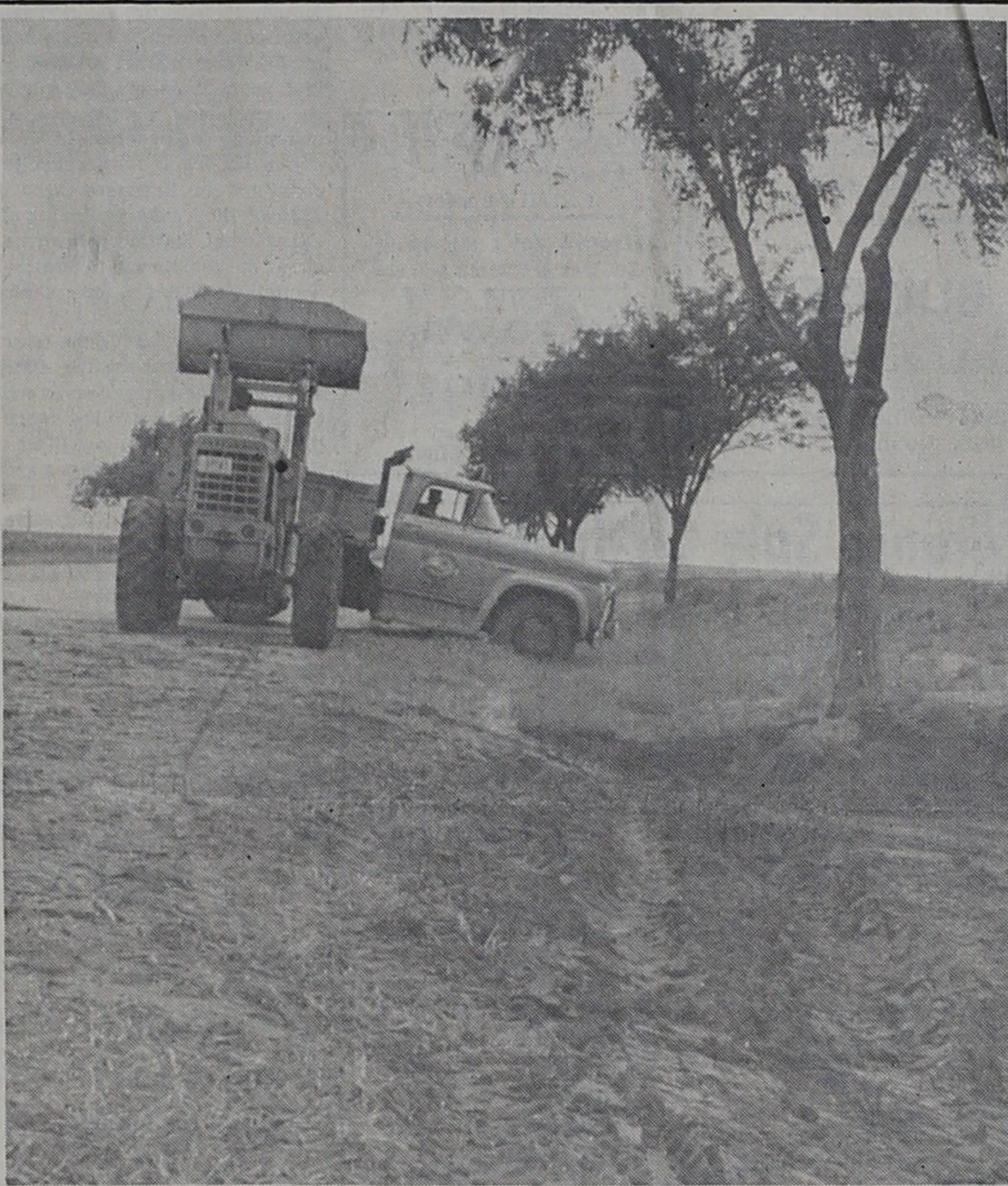
SCOOPING UP loads of what was formerly rich farm land, crews from the Highway Department dug out tons of rich soil from a highway barrow ditch last week. Some farmers were to use the soil for their lawns -- sort of expensive lawn dirt.
