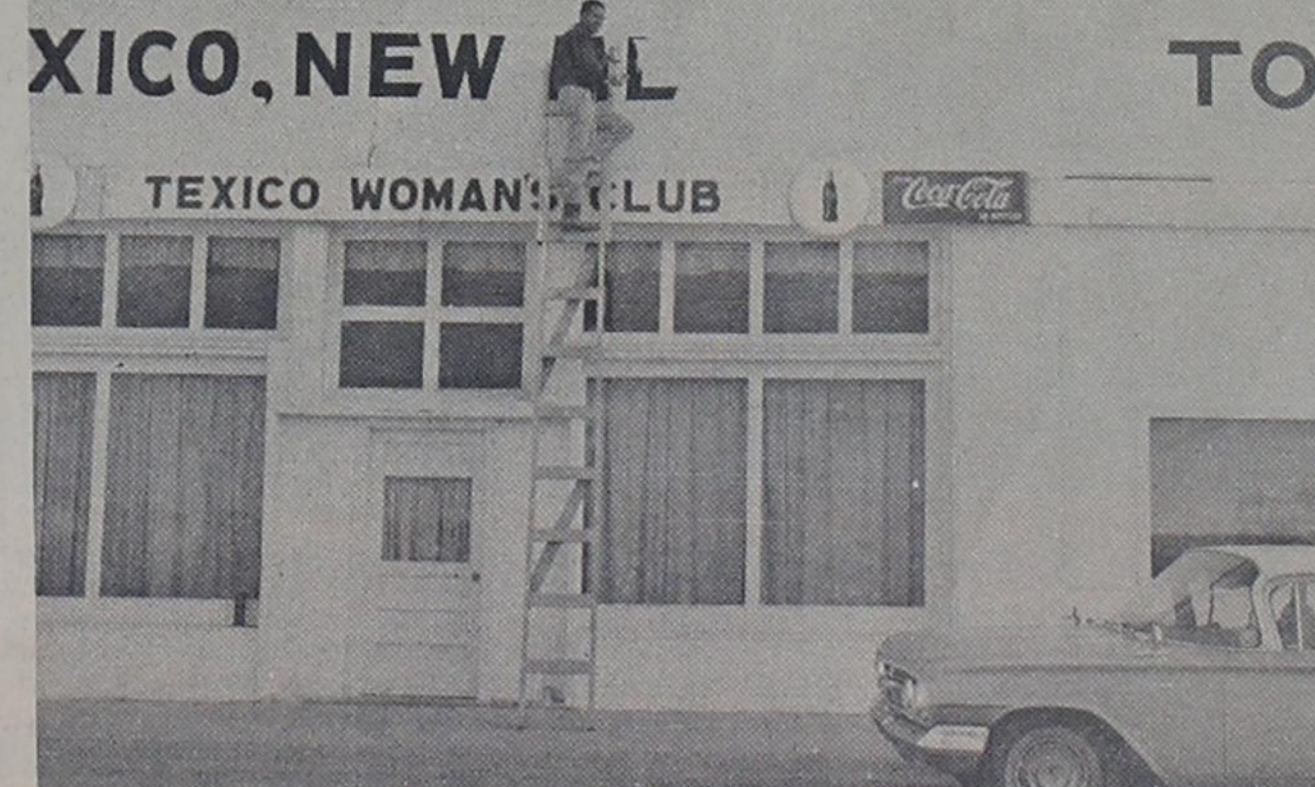
Calvin Young, Texico painter, is shown giving the town hall in Texico a face lifting. The block long area which houses the Woman's Club building, city offices and fire station are receiving a coat of white paint with the lettering in black.
