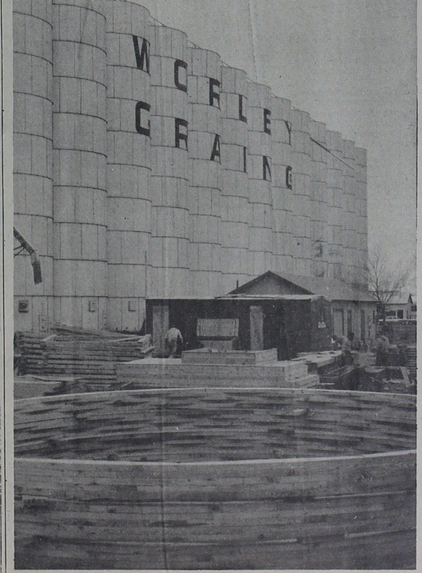
"SERIOUS WORK" IS BEGINNING at Worley Grain Company on their new concrete storage tanks which will add 300,000 bushels to the company's capacity. The circular wooden object in the foreground is a stack of forms that will be used to mold the circular concrete tanks.
