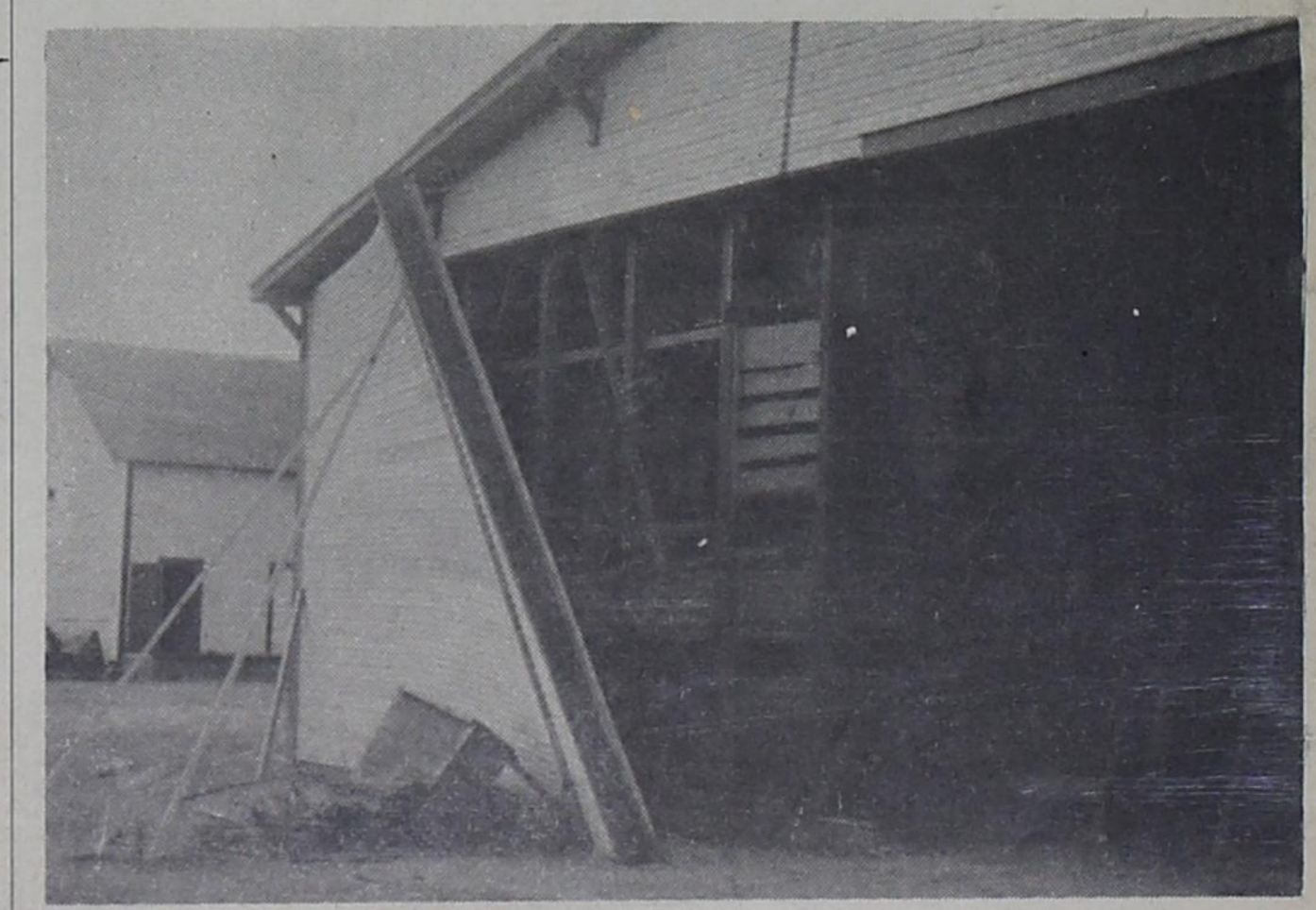
THE WIND REALLY BLEW--as evidenced by this picture taken at Kemp Lumber Wednesday. A 14-foot wall section on the east end of the large building was twisted away from the main structure Tuesday morning about 11. At noon, while personnel were out to lunch, the huge sliding door on the east end of the building blew down. Mrs. Joe Crume says, "It was the way the wind hit; it just twisted the wall away."
