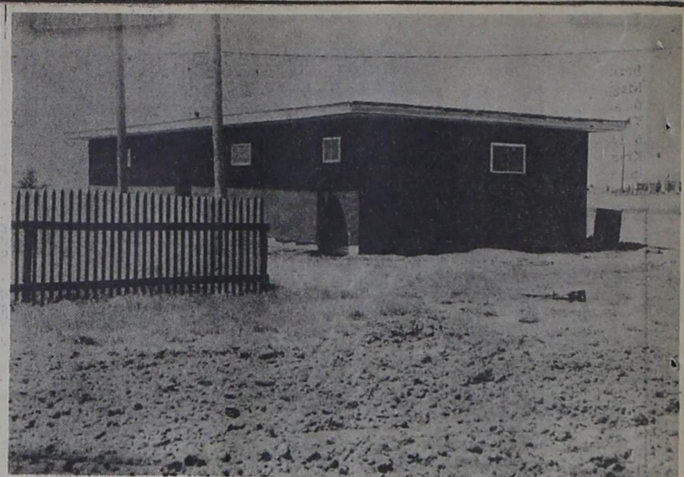
NEW MEETING ROOM for the Farwell fireboys is this half-completed frame building behind the fire hall. When Dale Berggren and his family moved into the apartment in the city hall, the fireboys had to look for other quarters. They decided to put up their own building, and volunteer labor, usually on the weekend, is getting the job done. Otis Huggins, fire chief, says the building will cost the department about $2,000.
