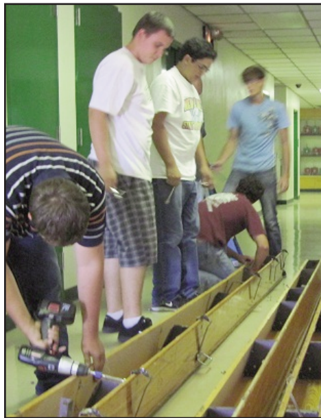
Dalton Wren, Eric Palaia, Matthew McWhorter, Mark Hughes, Tristan Lockmiller continue dis-assembly of bleacher sections. The classes salvaged all the wood and some of the usable steel for future projects.
