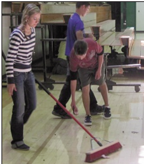
Audrey Wren, Logan Caselman, Haden Spears, Briana Reyna, and Brooks Hagler assist in dis-assembly of the old wooden bleachers in the gymnasium to make room for the new ones.
