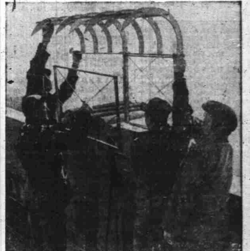
ANTI-SUICIDE PARAPET — Workers raise a section of the stainless steel parapet guard to be erected on the 86th floor observatory of the Empire State building, New York City, as a barrier to would-be suicides.
