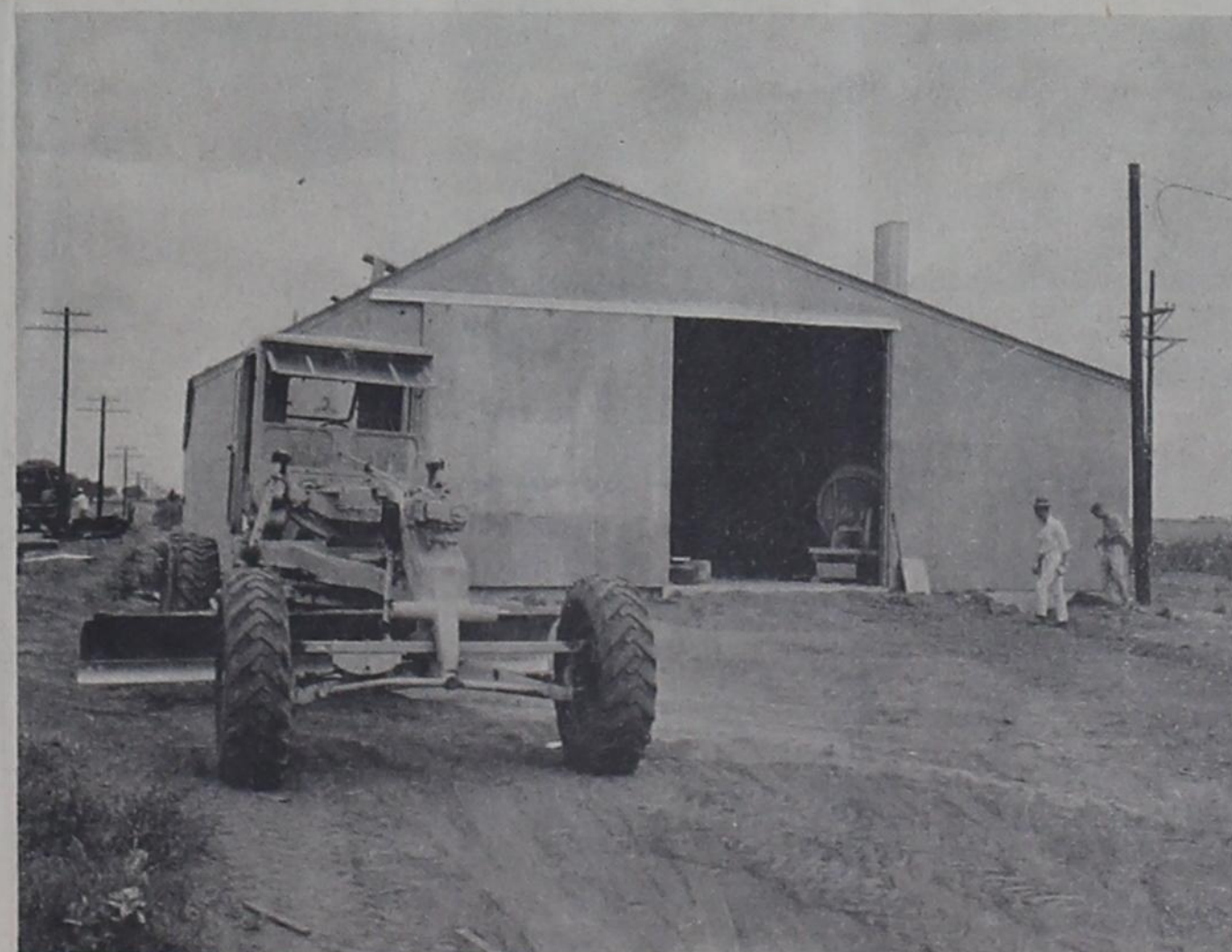
Work continues on the Monsanto Agricultural Center, east of Farwell. The plant is scheduled to open in the near future. Glenn Marsh is manager of the plant and Jimmy Walker is plant foreman.
