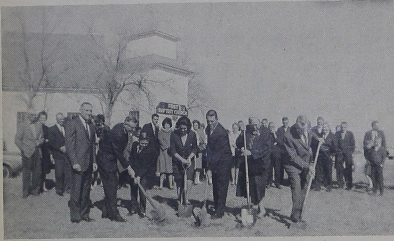
GROUND BREAKING -- Several members of Texico First Baptist Church along with Rev. Earl Landroop, Associational missionary, turned a shovel full of earth in unison Sunday (Jan. 3) at the groundbreaking ceremony for the new church building.
