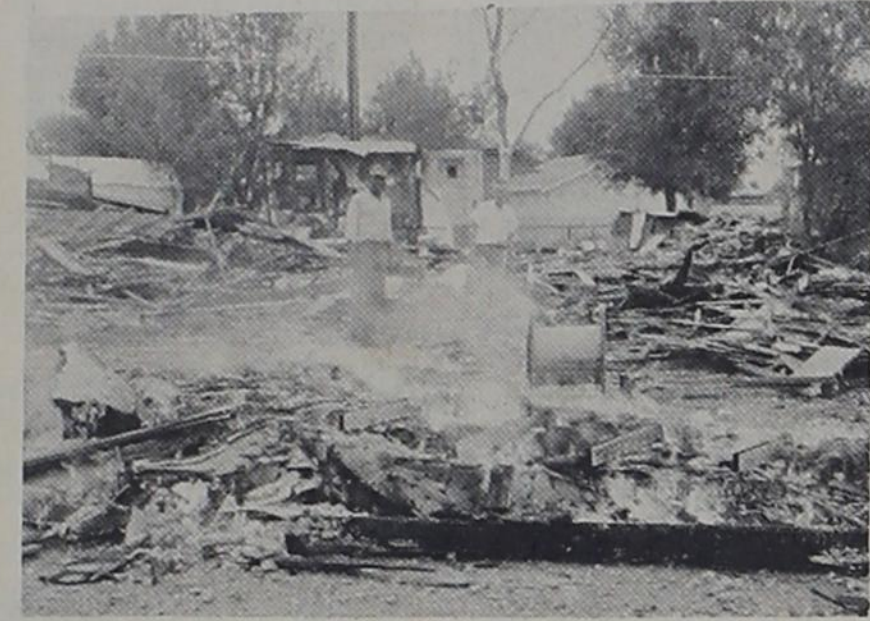
CLEANUP TIME -- Ray Stone, owner and operator of Village TV and Radio Shop, and Elbert Thomas were busy early this week cleaning up the piles of rubbish and charred lumber left at the former home of the company which was destroyed by fire recently. Local citizens interviewed in the recent Jaycee survey indicated that a general cleanup campaign in the towns would be of great benefit.
