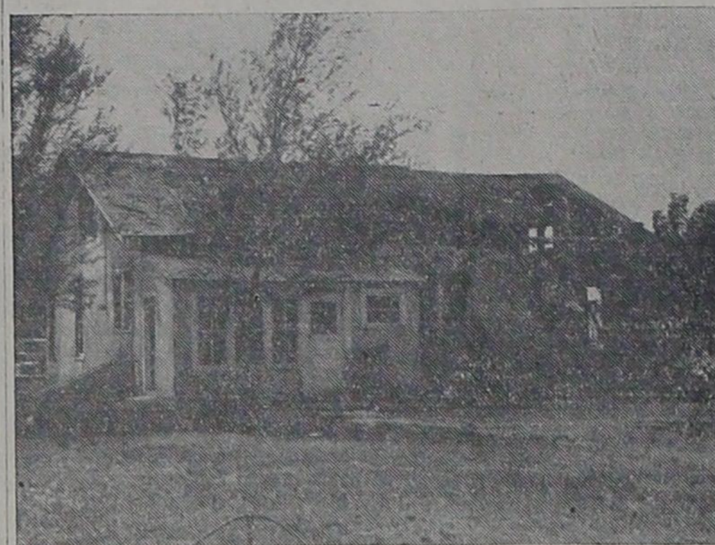
TERRIBLE FIRE —Very little was salvaged from the home of Mrs. Clytie Dial when fire struck Saturday evening. This is a view of the residence from the east, showing how the flames consumed most of the roof and gutted the building's interior.
