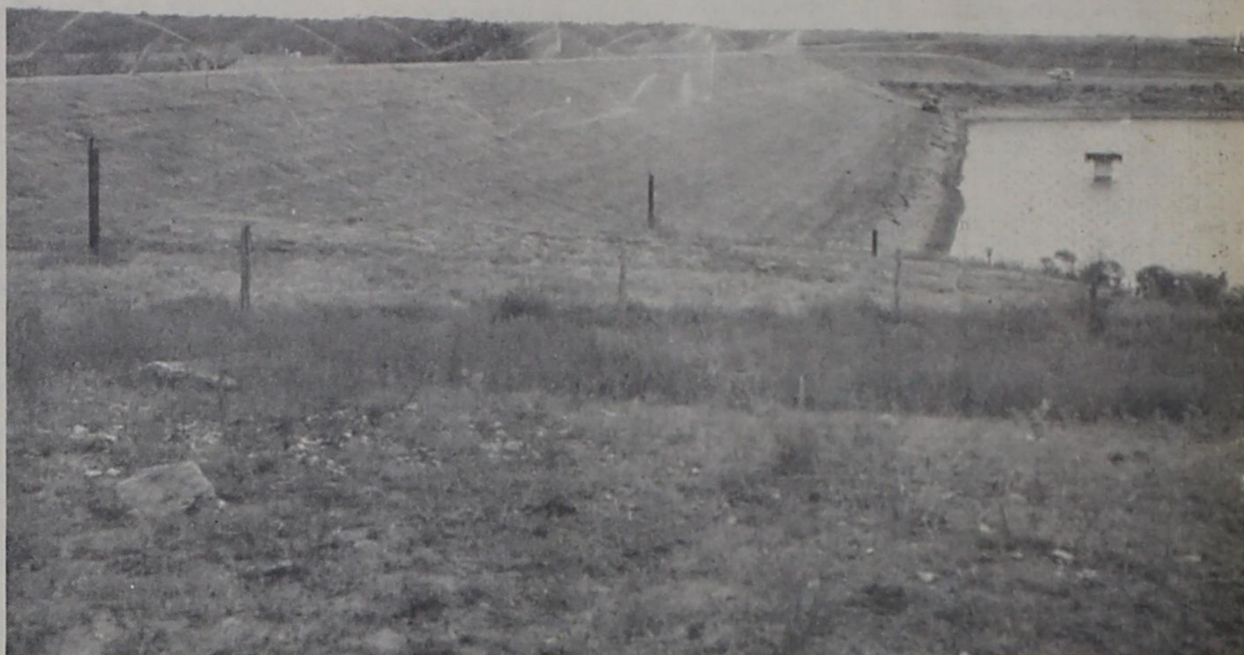
Irrigating Bermuda grass on a floodwater retarding structure by use of a sprinkler system pumping water from the lake area. This is the type of structures that are proposed for the Running Water Draw project. Note the draw-down tube to maintain a
