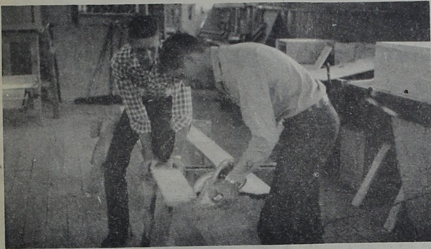
Pictured here is Ronnie and Lonnie Curry in the process of building a portable loading chute for their swine enterprise.
