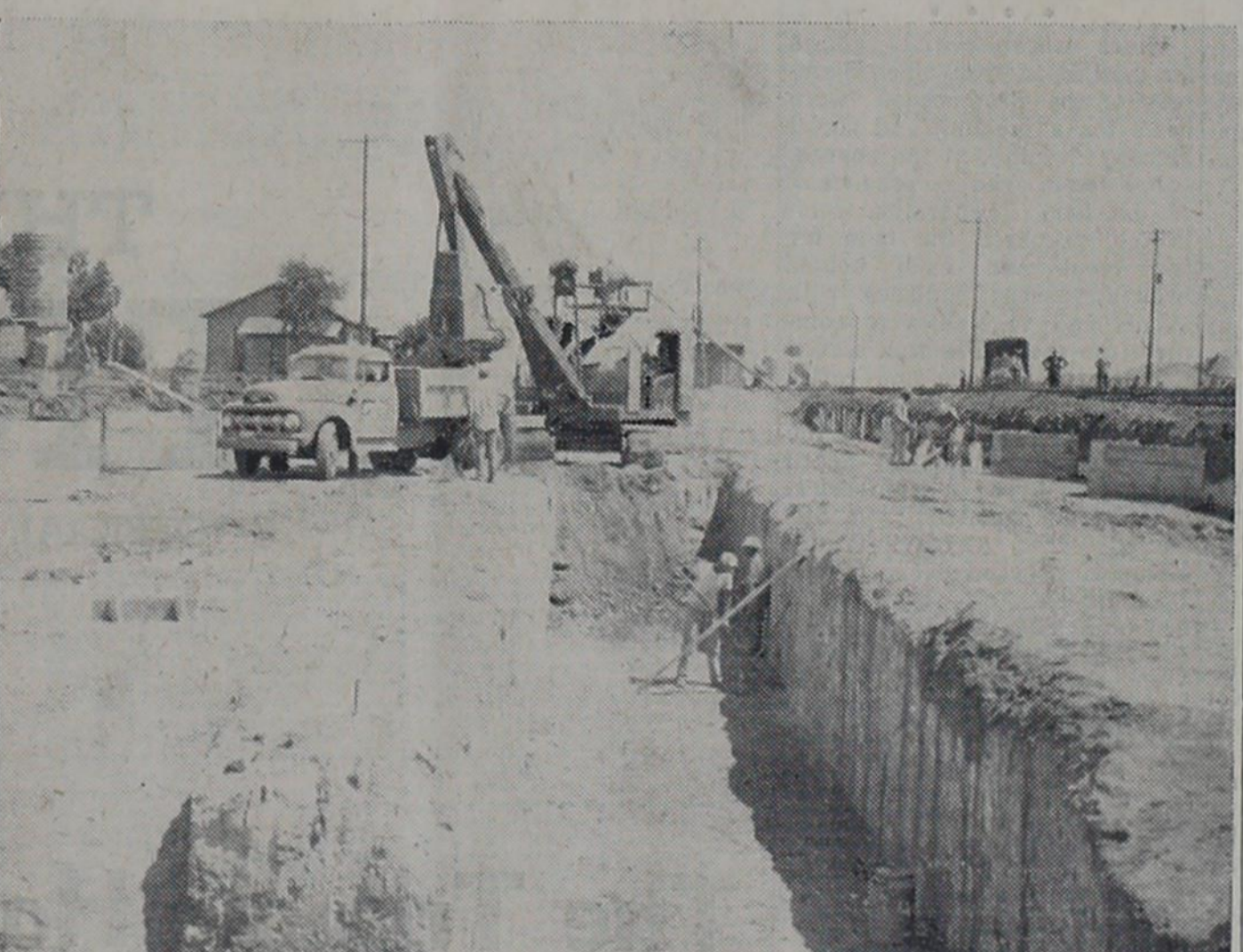
ELEVATOR GOING UP — Workmen conclude excavation work Monday afternoon on an expansion project at Sherley-Anderson Grain Company of Lariat. Pouring of concrete was to begin Tuesday on the 21 storage tanks which will increase the capacity of the elevator by 1,300,000 bushels. The project is scheduled to be completed in October.
