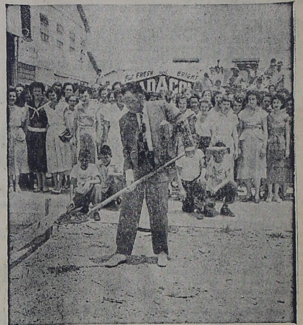
Senator Dudley J. LeBlanc, creator of famous HADACOL is shown above breaking ground for the new HADACOL factory now being built alongside the present plant in Lafayette, Louisiana. This new building will be 80x235 feet, two stories, steel and concrete construction. The remarkable growth of HADACOL has forced the immediate construction of this new building. Only last spring Senator LeBlanc opened the present HADACOL plant and now less than a year later, HADACOL requires a 100% increase in factory space.
