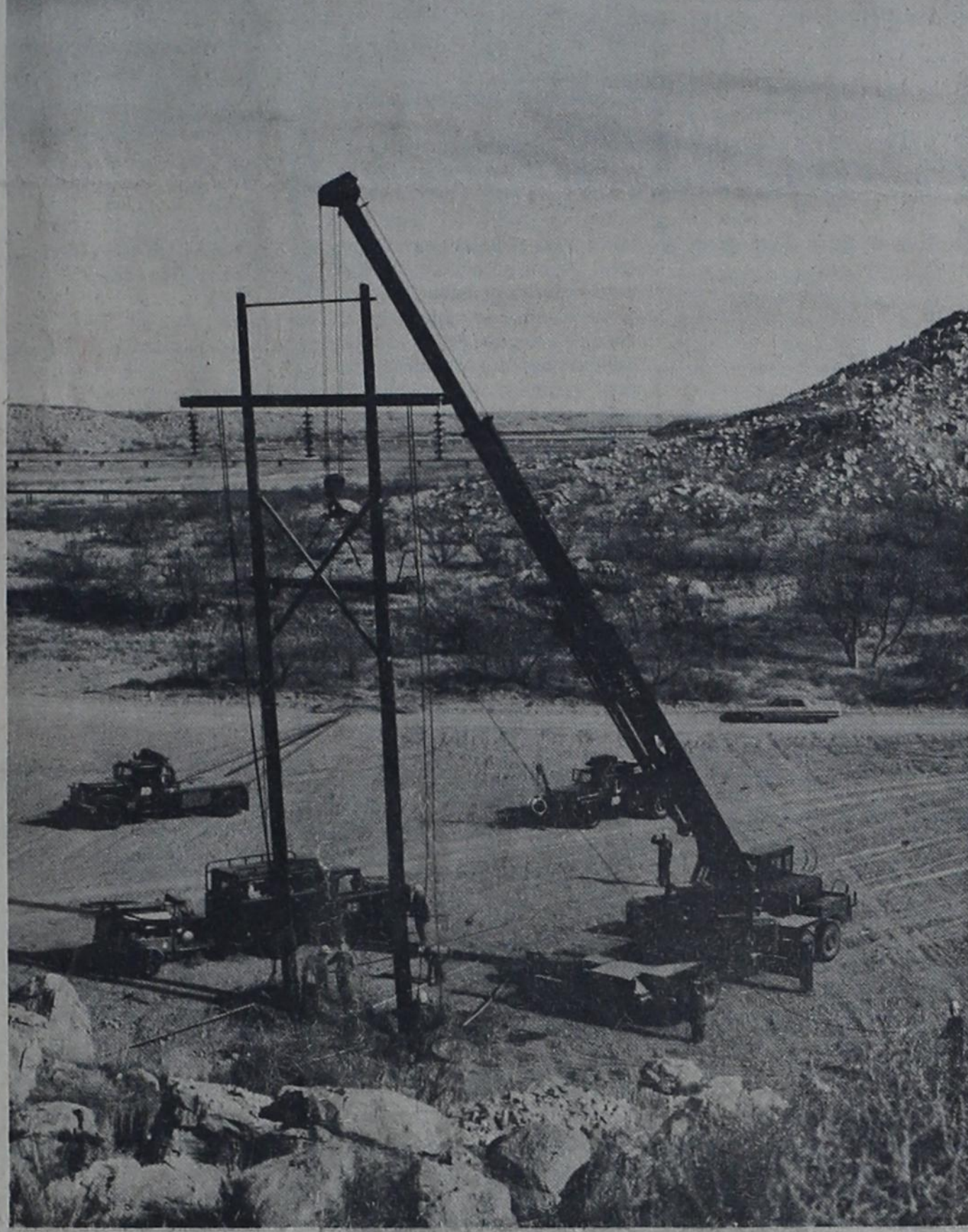
An 80 foot electric transmission line structure can be lifted and set into place in 8-1/2 minutes with Southwestern Public Service Company's new hydraulic crane. The unit, the second one to go into service in the nation, was specifically designed for use in the electric utility industry. Southwestern Public Service Company has announced a 1966 construction program calling for the investment of $19,353,000 in new facilities, with a large portion of the additional investment to be in transmission lines.
