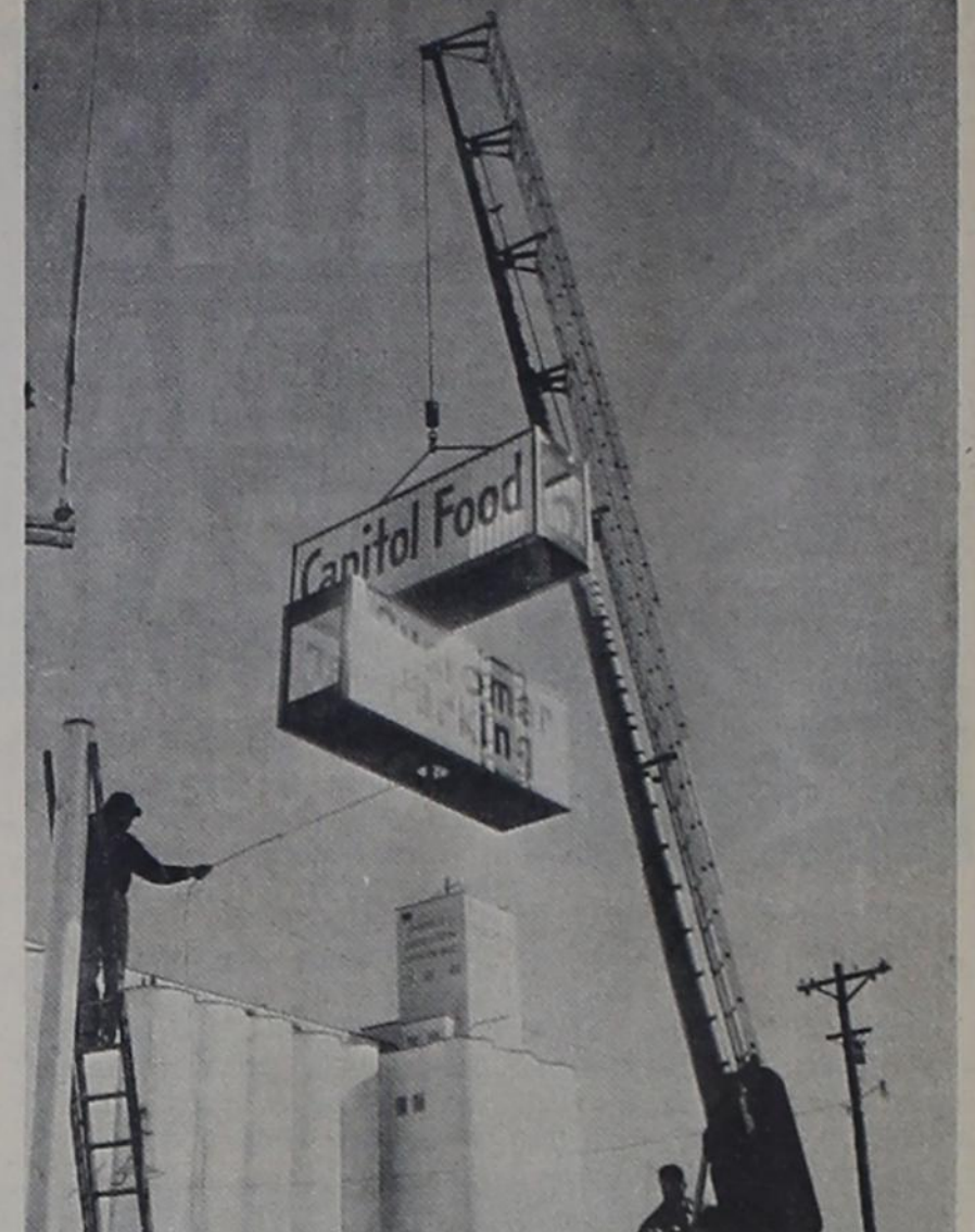
ALMOST READY ---Capitol Food Store in east Farwell is almost ready for the Grand Opening of their place of business scheduled for Feb. 1-6 with the installation of the huge neon sign which was being erected on Monday. The business opened in the new location early in December. Plenty of parking space is available for the customers on the paved parking area surrounding the store.
