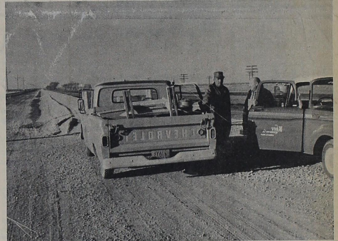
Joe Cope (left), superintendent of the 10.2 miles Parmer County highway project discusses the progression of the construction with Doc Brown, highway engineer. Caliche is ready for spreading over the new lane.
