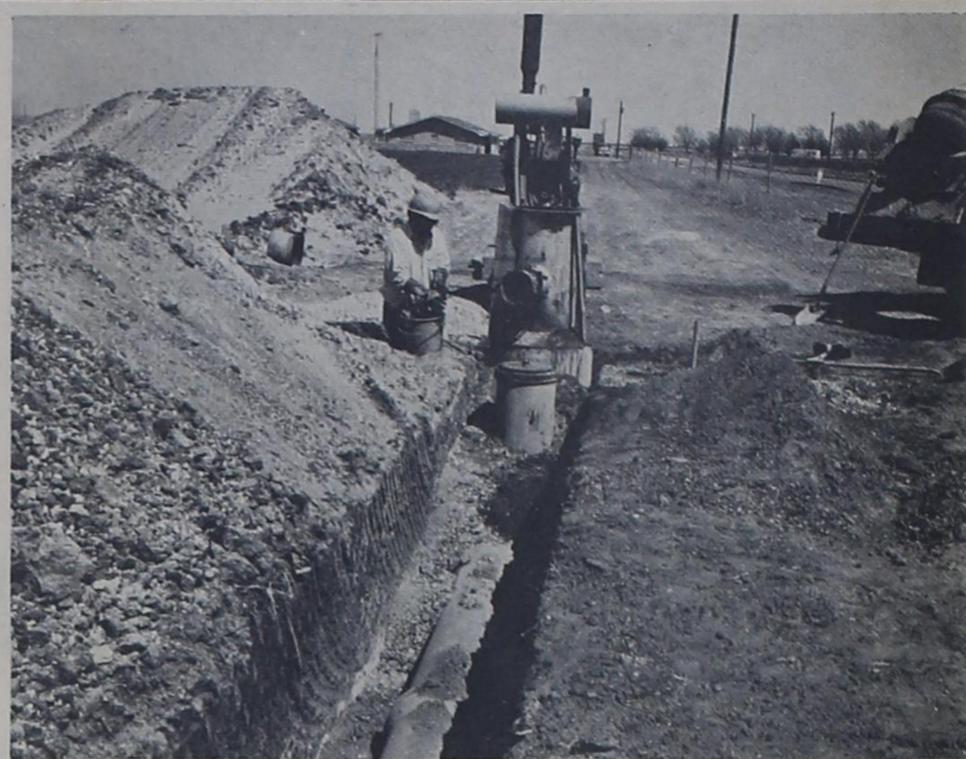
INSTALLING PIPELINE -- An underground concrete pipeline irrigation system is being installed on the Reagan Looney farm two miles southwest of Bovina. The system is designed to conserve irrigation water, Soil Conservationists say. (Photo by Jerry Isbell).
