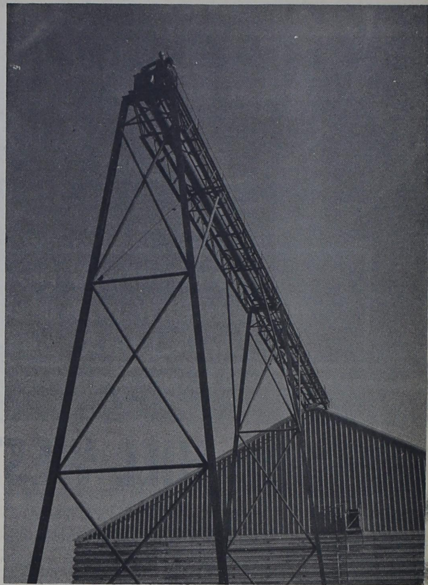
More grain storage is being built every year to handle the ever-increasing Farmer County production of wheat and grain sorghums and especially the latter. Here a workman is completing installation of an electric motor on an auger high above the ground near the just-completed West Friona Grain company.
