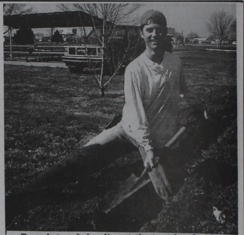
Ryan Autrey helps dig out the trenches for the new sprinkler system being installed at KKR Park in Texico.
