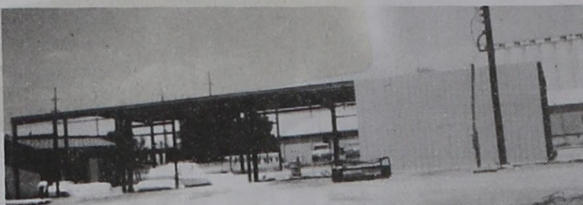
Business rebuilt Nathan "Butch" Tharp is having Triple Q Construction rebuild Tharp Dragline Service in Farwell. Heavy snows last winter knocked down part of the previous structure.
