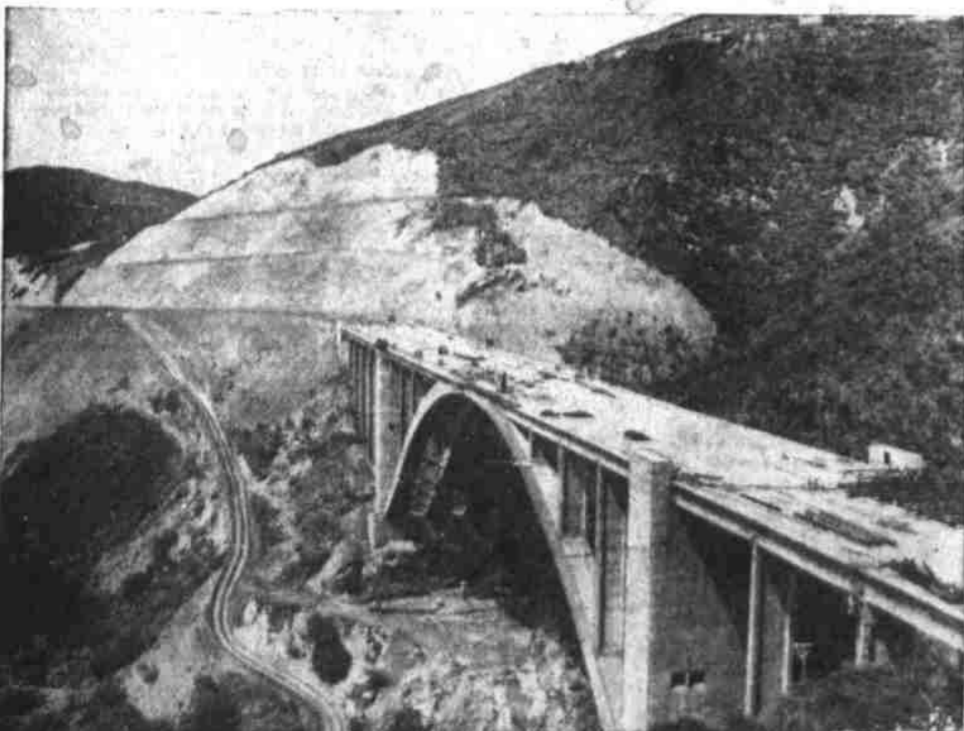
GOING ROUND THE MOUNTAIN — Work nears completion on pre-stressed concrete bridge between La Guaira and Caracas, Venezuela, in foothills of Andes. Bridge is 1,020 feet long, has 290-foot span 220 feet above creek and is one of longest of its type in world.
