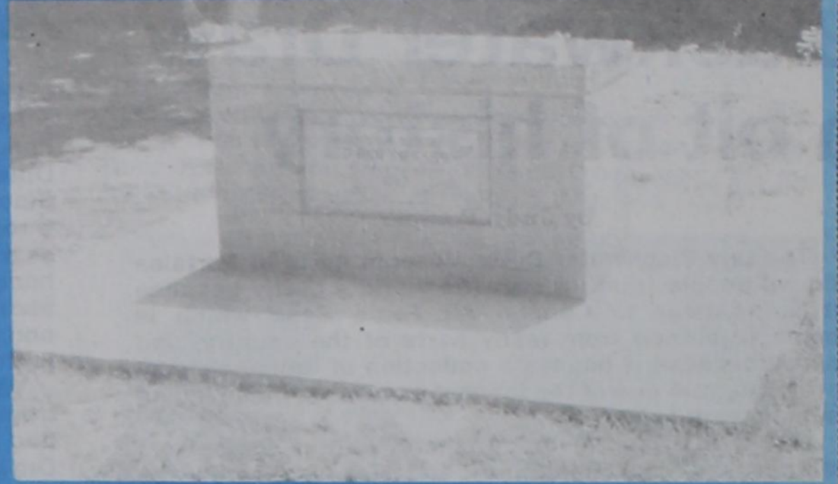
The masonry has been repaired on the drinking fountain at the Farwell Elementary School playground. It awaits the plumbing connection.
