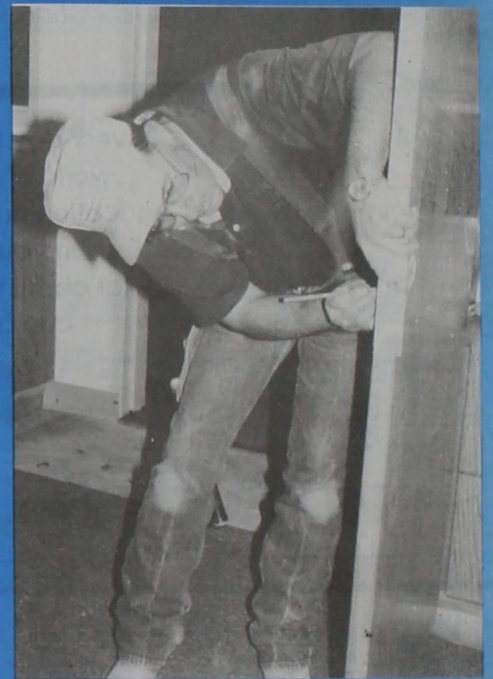
Herbie Hurst measures a door knob on a door in the new Junior High building.
