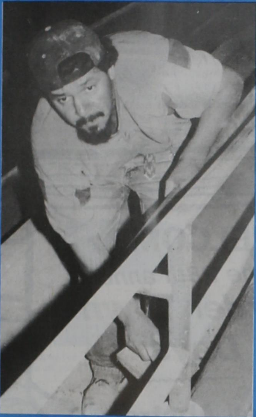
Chris Sena applies plaster under the guard rail in the new gym.
