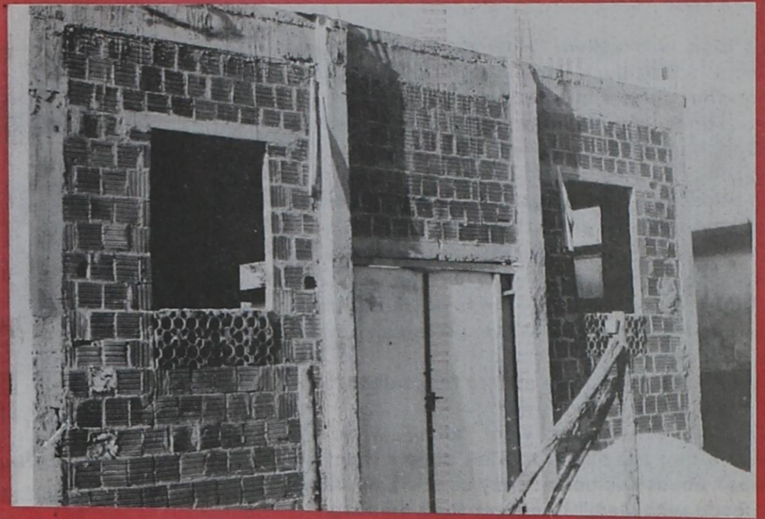
This building, Marco Dios, is not yet complete. Ciro and Yolanda Garcia and J. Grisham worked on it during this mission trip. Someday it may house a congregation.
