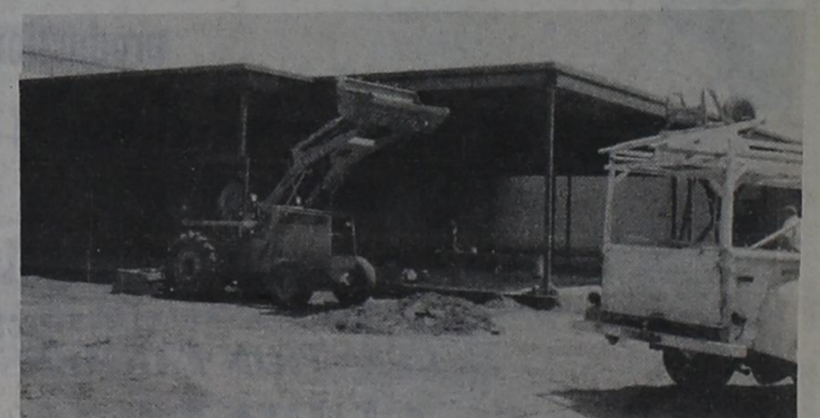
A bulldozer works on the new surgical unit at Clovis High Plains Hospital.
