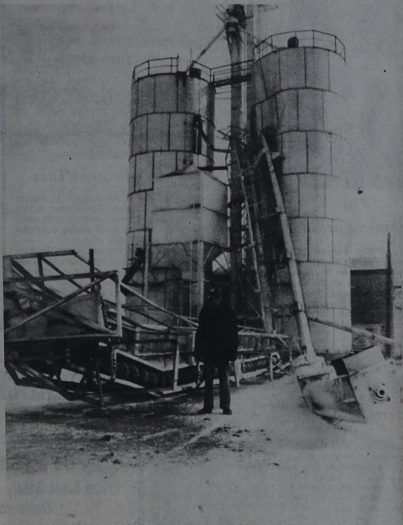
The legs on this grain elevator of Worley Mills Inc. in the Pleasant Hill community were blown down the evening of Thursday, Feb. 7, when winds reached velocities of 45 to 50
