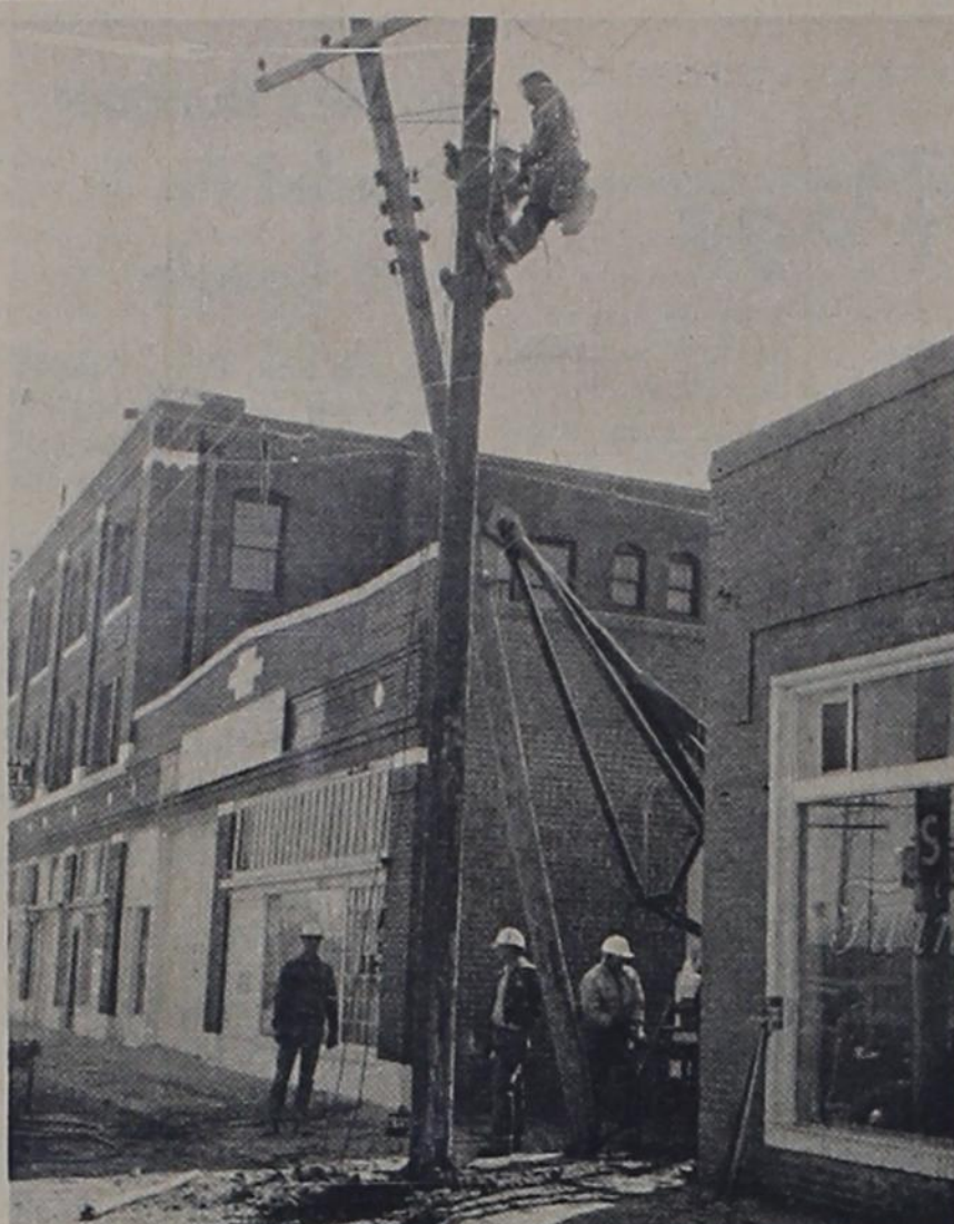
WORKMEN FOR SOUTHWESTERN PUBLIC SERVICE CO. replace a highline pole sheared off by a runaway trailer in the Texico business district Tuesday. No one was hurt.
