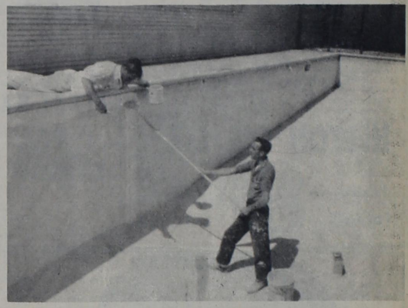
Workmen David and Zane Axe are shown here applying a fresh coat of paint to New-Tex swimming pool. The pool is scheduled to open at 1 pm today.
