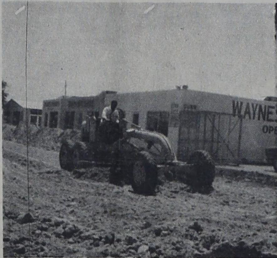
The parking areas in front of these businesses in east Farwell are getting face-lifting job this week. A construction crew was busy leveling ground in preparation for paving which will be in front of Wayne's Supermarket, Hughes Auto Parts, Farwell Plumbing and Live Longer Laundry. The project is hoped to be completed by the end of the week.
