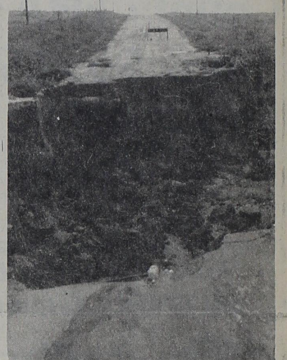
FLOOD WATERS WASHED OUT this road north of the Pleasant Hill community near Frio Draw. The washed-out area was about 15 feet in depth and 30 feet across. This area received nearly 10 inches of rain in one 24-hour period.
