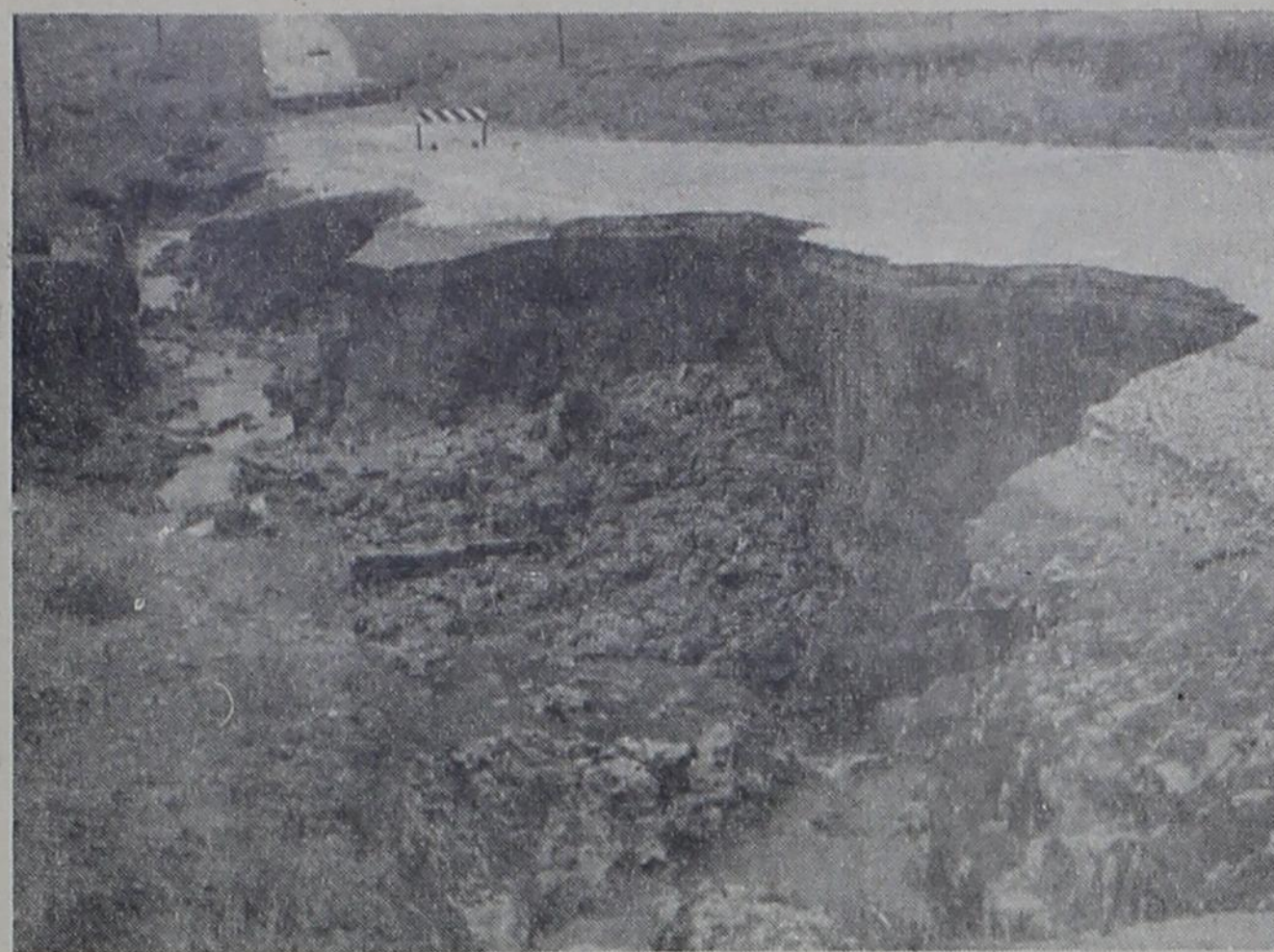
PART OF PAVED STATE LINE ROAD north of Pleasant Hill was washed away during the downpour. Further down the road (just off the pavement) is where the complete road was washed away. Beyond the next hill is Frio Draw.
