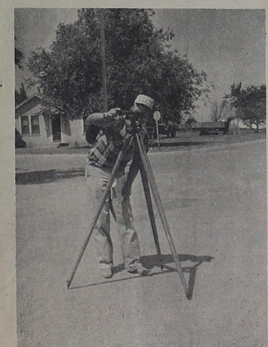
BEFORE THE PAVING can be installed in Farwell's new improvement project surveying must be done to establish grades. Here a surveying instrument is in use on Avenue B. The project is "ready to roll" and construction will begin immediately.
