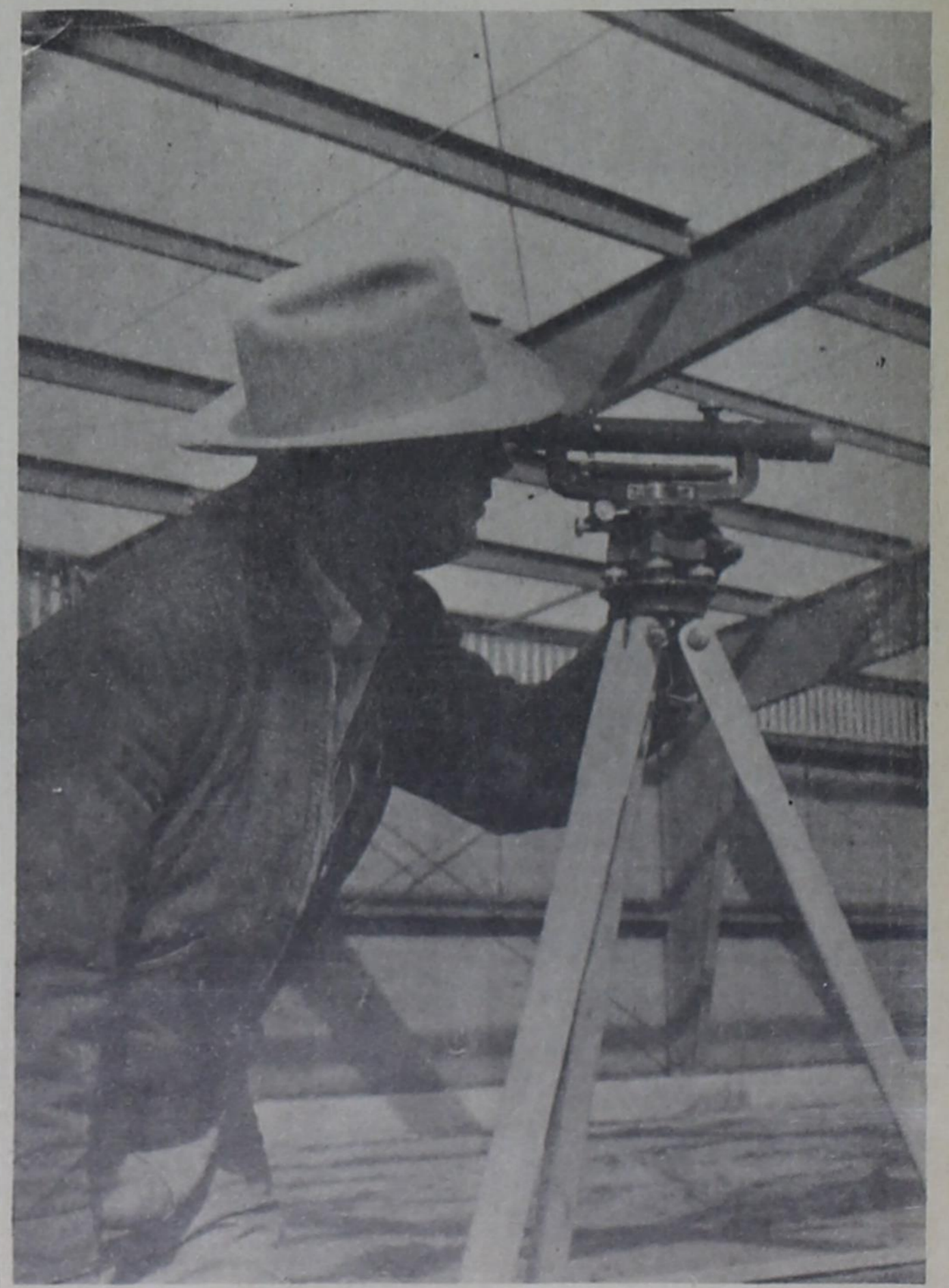
SIGHTING "ER IN--E. E. Hooper of Dura-Bilt Products, Clovis, takes a look through a level to check grades on flooring being run in the new A-A Bowling Lanes building now under construction in East Farwell. A very cold winter has held up work on the building drastically, although sheet steel has been applied to the walls of the framework.
