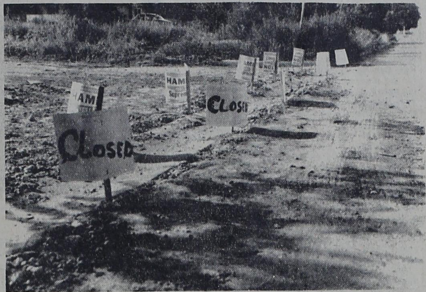
GET THE MESSAGE? The marking of this new curbing on Third Street is a John Aldridge project. The resourceful attorney used old political placards as warning signs for motorists to keep off the curing concrete. "It'll take a terrible driver to knock all those signs down," predicted Aldridge.
