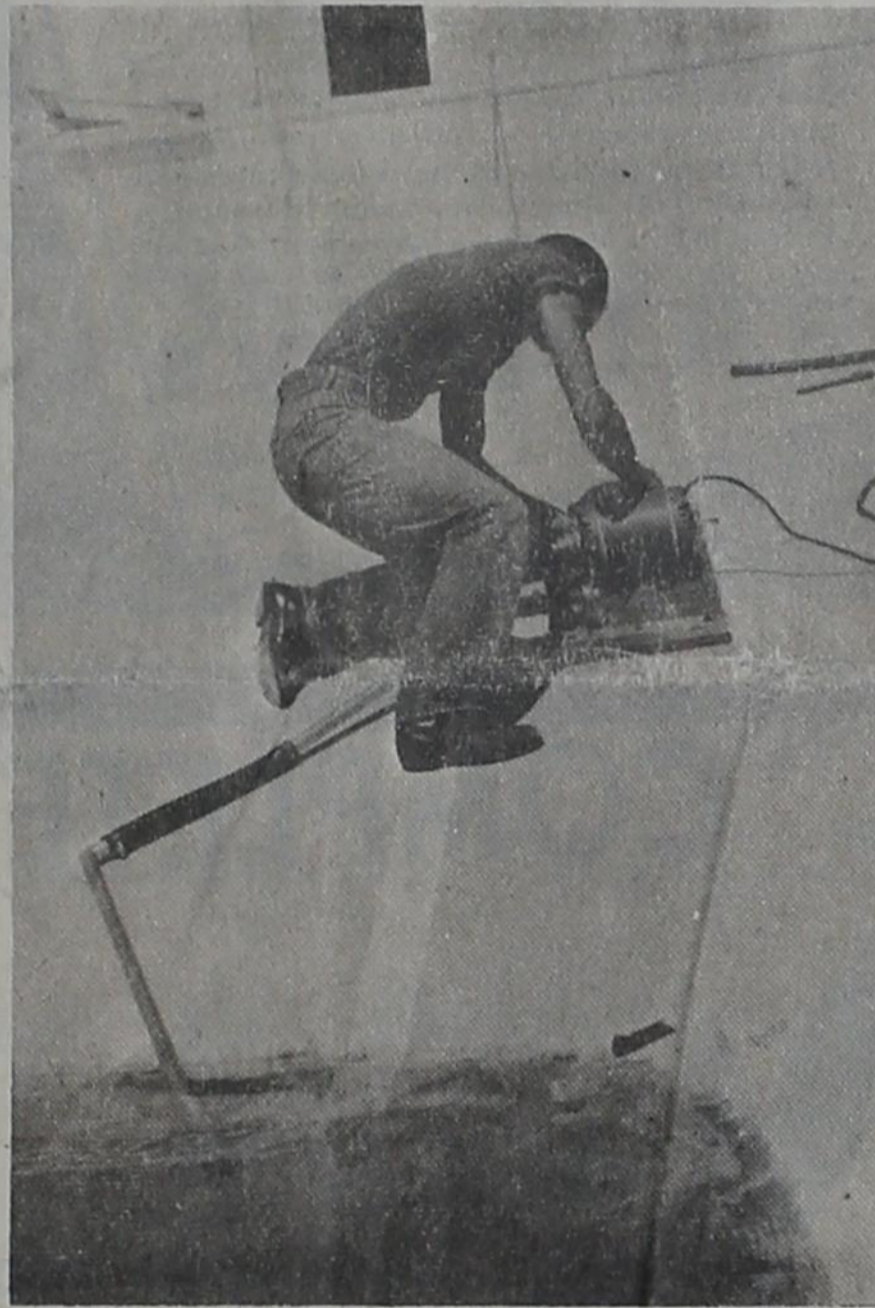
SLU-R-R-P, and the dirty rainwater from the new swimming pool is sucked up over the side. Jerry Henson, pool manager, here adjusts a centrifugal pump that will remove the unwanted water. The pool operators didn't want to unplug the drain in the bottom of the pool because sand and other debris might clog the mechanism. Riley Boss loaned them this small electric pump.
