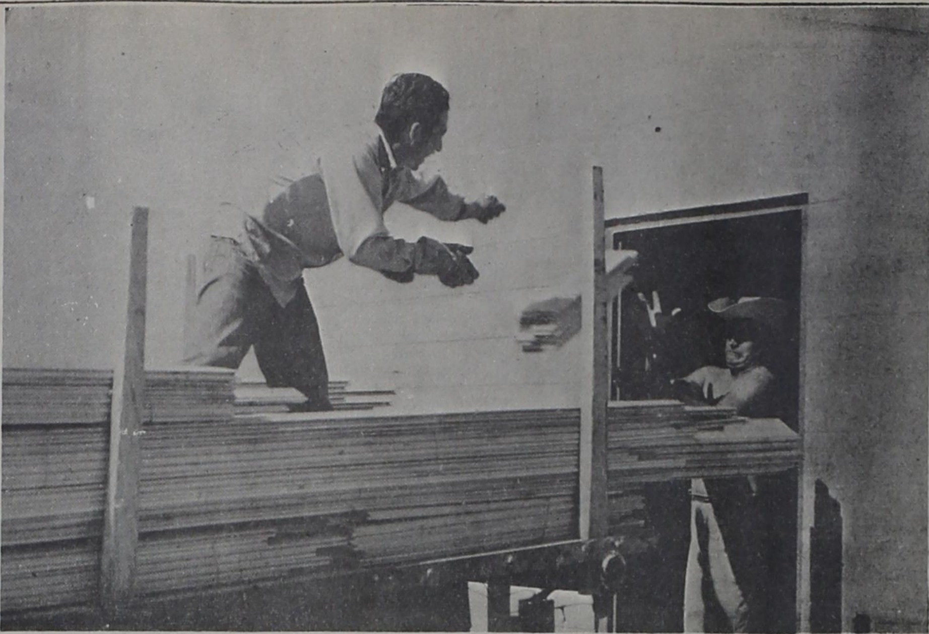
WATCH OUT, JOSE!--A workman grimaces as he readys himself for a catch of a batch of hardwood flooring being loaded into Meeks' new roller rink. Insulation of the building has recently been finished, and the laying of the floor will bring the project almost to completion.
